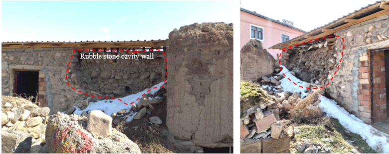
Figure 11. The outer rubble stone wall delamination in Malatya
