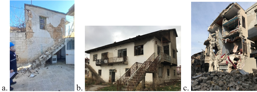
Figure 6. a. A damaged masonry 2-floor village house in Nizip, Gaziantep b. Slightly damaged masonry house in the city center of Elbistan, Kahramanmaraş c. Extensive partial collapse of a masonry 4-floor building in Antakya, Hatay city center.
