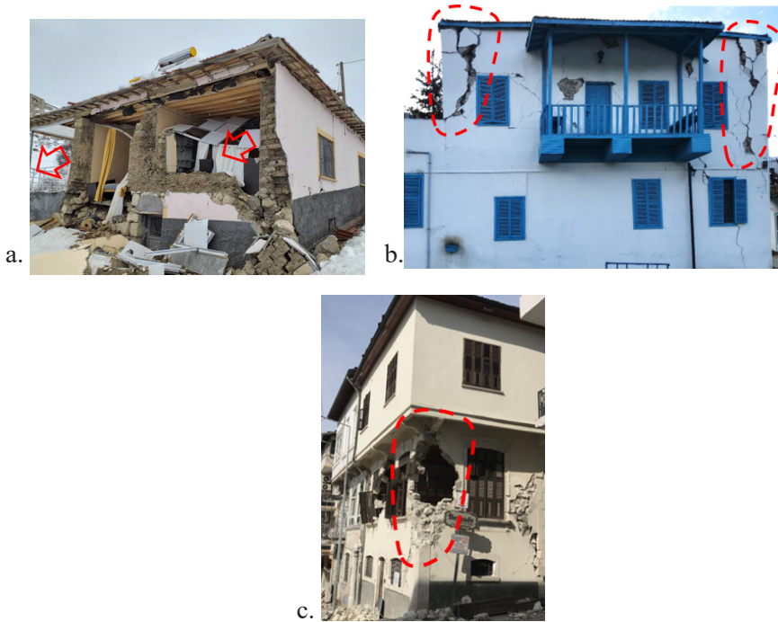
Figure 15. a. Wall-to-wall connection failure b. Corner failure along with in-plane damages c. Partial collapse due to lack of corner connection and in-plane damages
