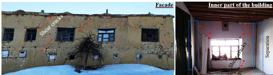
Figure 7. Shear cracks within the plane of masonry walls, coupled with separation.
