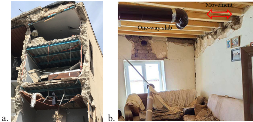
Figure 13. a. Slab-to-wall connection failure b. Inappropriate anchorage of timber joist in adobe masonry
