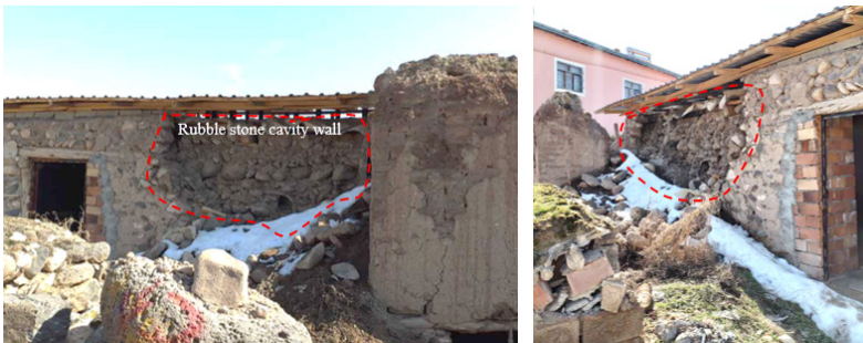
Figure 11. The outer rubble stone wall delamination in Malatya
