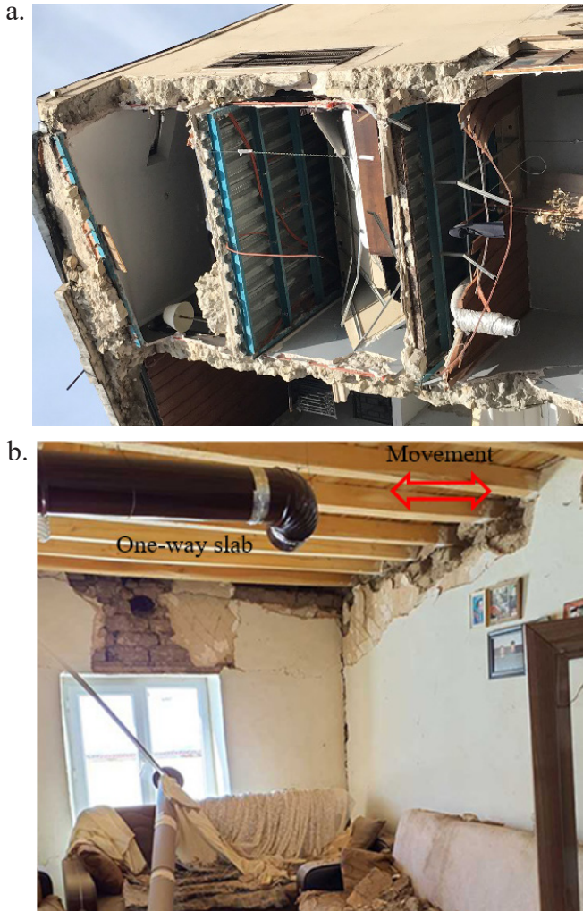
Figure 13. a. Slab-to-wall connection failure b. Inappropriate anchorage of timber joist in adobe masonry
