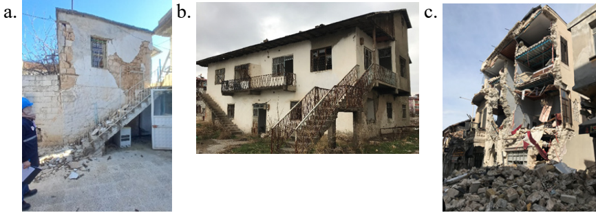
Figure 6. a. A damaged masonry 2-floor village house in Nizip, Gaziantep b. Slightly damaged masonry house in the city center of Elbistan, Kahramanmaraş c. Extensive partial collapse of a masonry 4-floor building in Antakya, Hatay city center.
