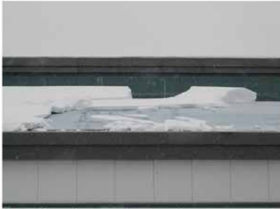
Sliding snow from a roof step on a smooth membrane roof. Photo Credit: Northern Microclimate Inc.
