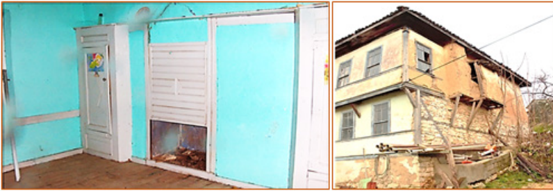
Figure 20. Hearth and Gusulhane extensions in the room on the main floor and overhangs to the garden
