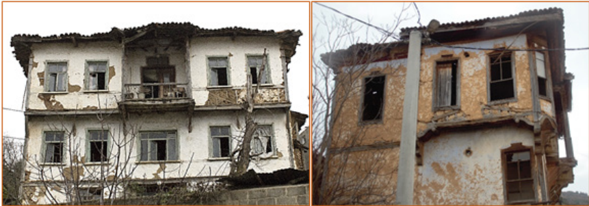
Figure 37. Examples of neglected and dilapidated houses
