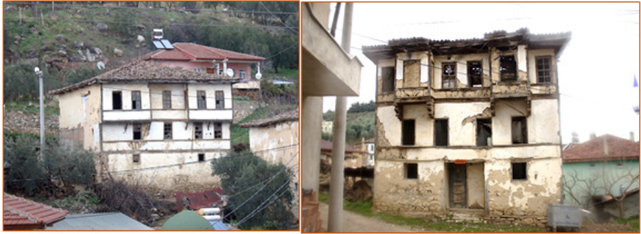
Figure 7. Examples of houses belonging to the Ottoman period in the Inikli local housing texture, which are not in use today and remain in a dilapidated state
